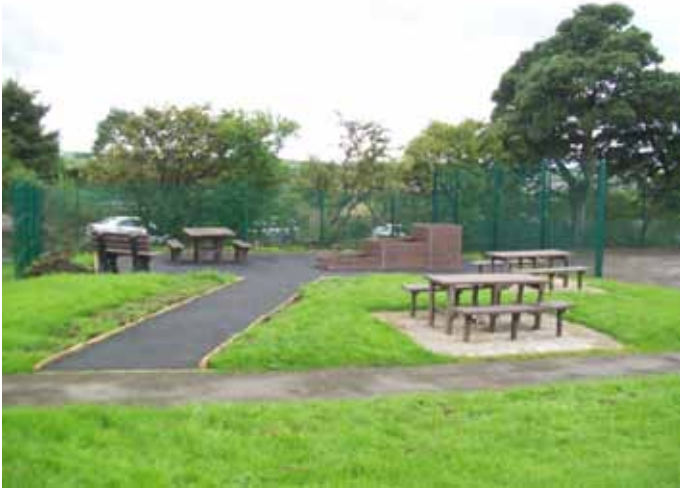
Fig. 17 Work in progress on a large project developing a sensory garden at Broadfield Specialist School
